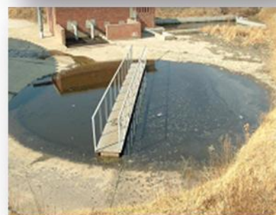
Advanced state of disrepair of the Petrus Steyn plant - primary settling tanks overflowing and blocked; deteriorated ponds.
